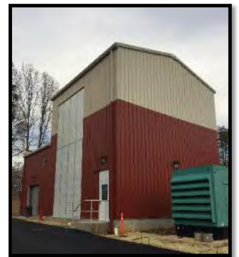
North Rivanna WTP 1 Contactor 40,000 pounds of GAC 1 MGD Capacity
