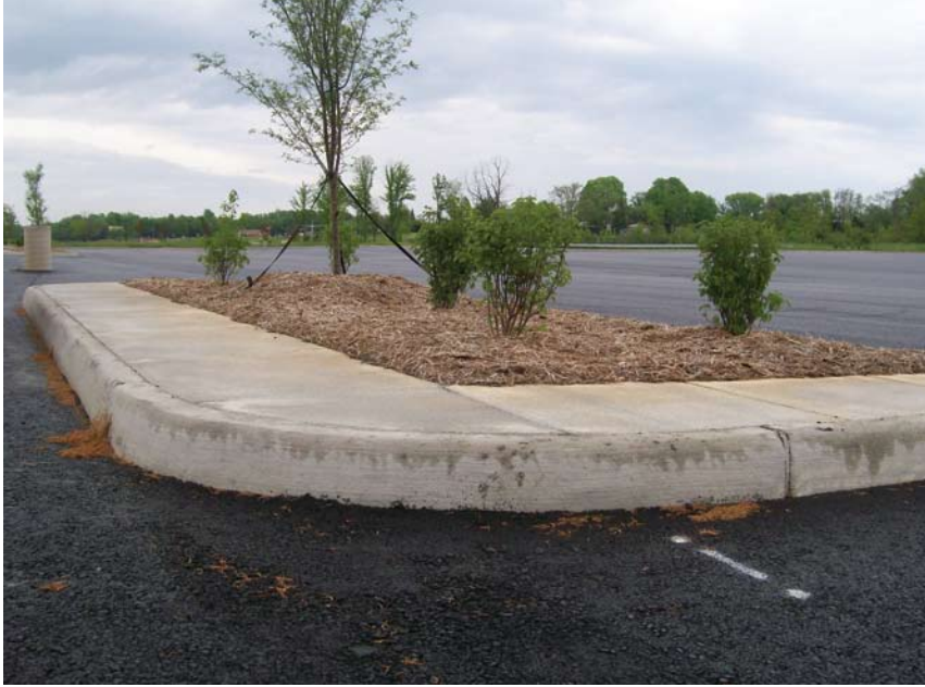
Raised islands such as this provide landscaping, but relatively little stormwater treatment.
