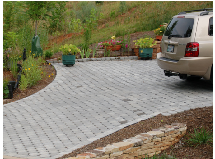
Porous pavers allow rainwater to percolate be absorbed into the ground below. A few recent projects in our area have incorporated them for parking areas and driveways, like the RiverBluff development in Charlottesville.
