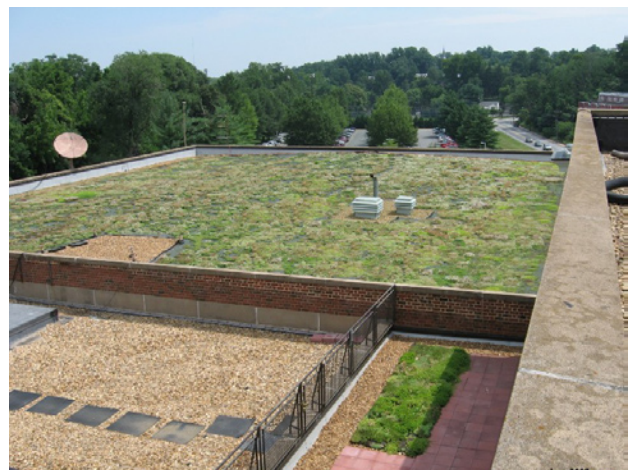
An excellent example of a green roof can be found on the Albemarle County office building located on McIntire Road.
