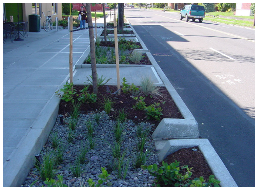
Periodic curb cuts allow some street runoff to drain into planting areas like the ones pictured in the example above.
