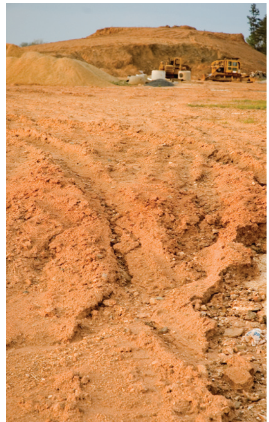
Development sites in the County too often resemble barren “moonscapes,” completely stripped of trees and plants that could help slow and filter runoff.
